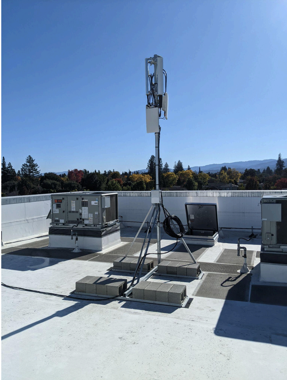
As of the 2023-2024 school year, each active school campus has this same radio setup to provide network coverage. Where possible the radios are mounted on the highest building on campus.
