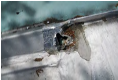
Typical Deficiency - Roof transition is open. Recommend removal of all temporary repairs and installation of as needed permanent repairs.
