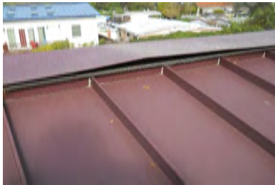
Typical Deficiency - Ridge cap has buckled. Recommend removal and reinstallation incorporating an expansion plate for movement.
