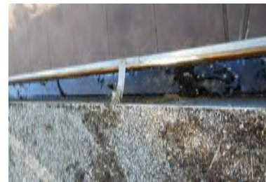
Typical Deficiency - Gutters are full of debris. Recommend clearing debris from all gutters, drains, waterways, and field of roof to promote positive drainage.
