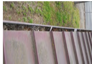
Typical Deficiency - Gutters are full of debris. Recommend clearing debris from all gutters, drains, waterways, and field of roof to promote positive drainage.
