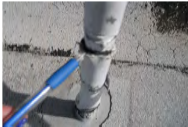
Typical Deficiency - Through roof penetration has not been properly sealed. Recommend re-sealing and installing storm collar.
