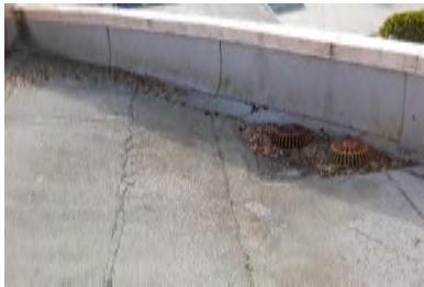
Typical Deficiency - Debris have accumulated at field of roof. Recommend clearing debris from all gutters, drains, waterways, and field of roof to promote positive drainage.
