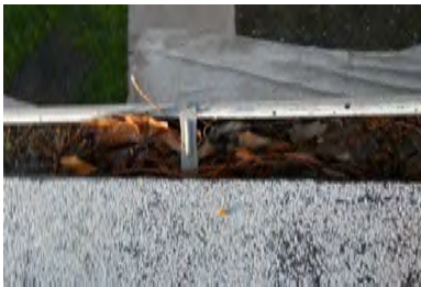
Typical Deficiency - Gutters are full of debris. Recommend clearing debris from all gutters, drains, waterways, and field of roof to promote positive drainage.
