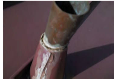
Typical Deficiency - Pipe jacks are missing sealant. Recommend application of flexible flashing self-adhered tape and or sealant, and install storm collar.
