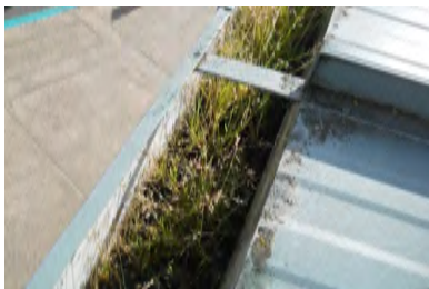
Typical Deficiency - Gutters are full of debris. Recommend clearing debris from all gutters, drains, waterways, and field of roof to promote positive drainage.
