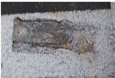
Typical Deficiency - Mineral surfaced cap sheet is damaged from previous sleeper block that has been removed. Recommend repairing as needed.
