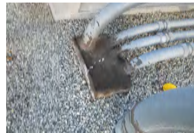
Typical Deficiency - Pitch pocket sealants have dried out and pulled away from flashing. Recommend topping off pitch pocket with compatible sealer or modified mastic and application of acrylic or silicone coating to preserve and maintain repair.
