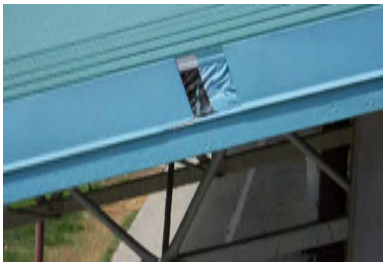
Typical Deficiency - Metal fascia detail is incomplete. Recommend repairing as necessary to provide a water tight application.
