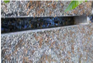
Typical Deficiency - Gutters are full of debris. Recommend clearing debris from all gutters, drains, waterways, and field of roof to promote positive drainage.
