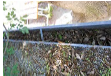
Typical Deficiency - Gutters are full of debris. Recommend clearing debris from all gutters, drains, waterways, and field of roof to promote positive drainage.
