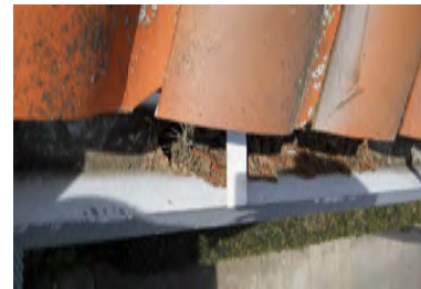
Typical Deficiency - Gutters are full of debris. Recommend clearing debris from all gutters, drains, waterways, and field of roof to promote positive drainage.
