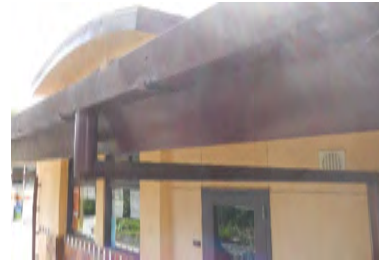
Typical Deficiency - Damaged gutter. Recommend repair as needed.
