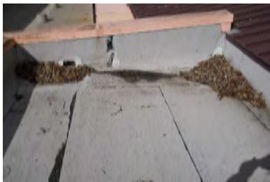
Typical Deficiency - Debris have accumulated at field of roof. Recommend clearing debris from all gutters, drains, waterways, and field of roof to promote positive drainage. Through wall scuppers should have debris screens. Recommend installation of gutter screens to promote positive drainage.
