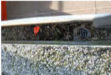
Typical Deficiency - Gutters are full of debris. Recommend clearing debris from all gutters, drains, waterways, and field of roof to promote positive drainage.
