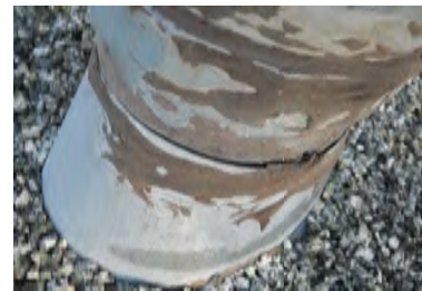
Typical Deficiency - Detailing at through roof penetrations show signs of cracking and delamination. Recommend touch up of mastic at penetrations and application of acrylic or silicone coating to preserve and maintain repair.
