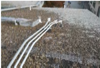
Typical Deficiency - Debris have accumulated at field of roof. Recommend clearing debris from all gutters, drains, waterways, and field of roof to promote positive drainage.
