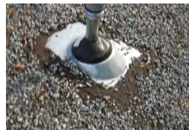
Typical Deficiency - Through roof penetrations do not appear to have proper roof jack. Recommend installing proper roof jack and storm collar.
