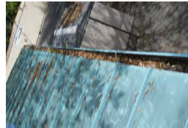
Typical Deficiency - Gutters are full of debris. Recommend clearing debris from all gutters, drains, waterways, and field of roof to promote positive drainage.
