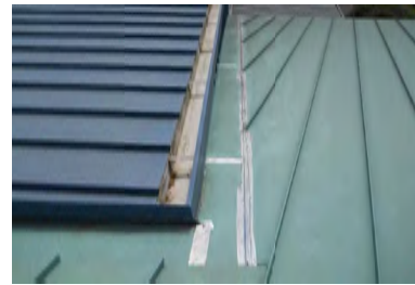
Typical Deficiency - Roof transition/ cricket has been temporarily sealed. Recommend removal of all temporary repairs and installation of as needed permanent repairs.
