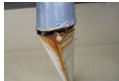
Typical Deficiency - Leader pipe seam is broken. Recommend repairing and or replacement.
