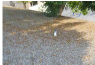
Typical Deficiency - Debris have accumulated at field of roof. Recommend clearing debris from all gutters, drains, waterways, and field of roof to promote positive drainage.
