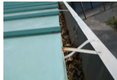
Typical Deficiency - Gutters are full of debris. Recommend clearing debris from all gutters, drains, waterways, and field of roof to promote positive drainage.
