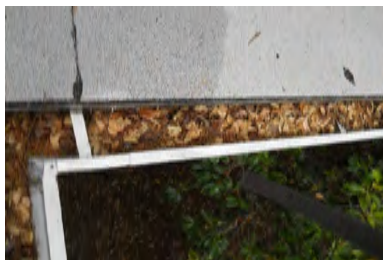
Typical Deficiency - Gutters are full of debris. Recommend clearing debris from all gutters, drains, waterways, and field of roof to promote positive drainage.
