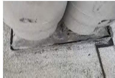
Typical Deficiency - Pitch pocket sealants have dried out and pulled away from flashing. Recommend topping off pitch pocket with compatible sealer or modified mastic and application of acrylic or silicone coating to preserve and maintain repair.
