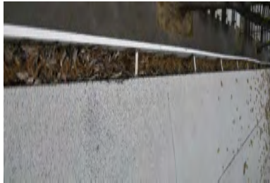
Typical Deficiency - Gutters are full of debris. Recommend clearing debris from all gutters, drains, waterways, and field of roof to promote positive drainage.
