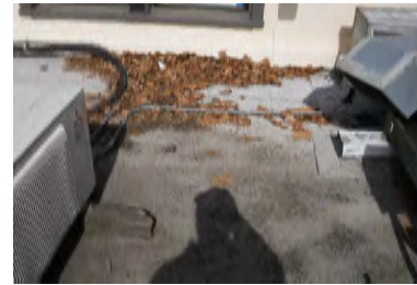
Typical Deficiency - Observed debris at field of roofing. Recommend clearing debris from all gutters, drains, waterways, and field of roof to promote positive drainage.
