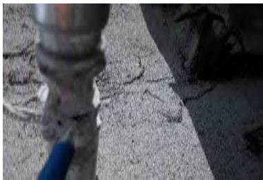
Typical Deficiency - Pipe jacks are missing sealant. Recommend application of flexible flashing self-adhered tape and or sealant, and install storm collar.
