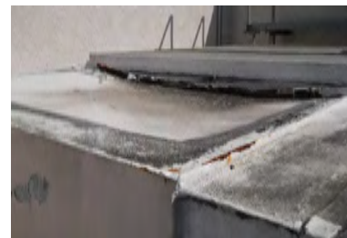
Typical Deficiency - Mechanical duct work damaged and deteriorated. Recommend replacement of damaged duct by licensed mechanical contractor and coating with acceptable silicone or acrylic coating.
