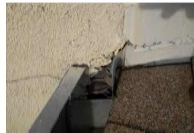
Typical Deficiency - Observed exposed lath and underlayment at roof to wall transition. Recommend stucco patch and as needed sealing to protect underlayment and minimize water intrusion behind stucco.
