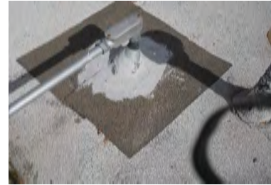
Typical Deficiency - Through roof penetrations has not been properly flashed. Recommend installing new roof jack and storm collar.
