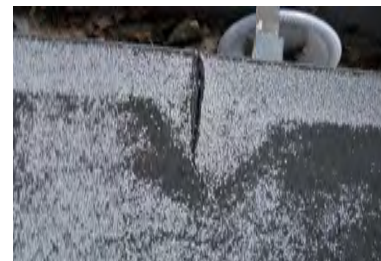
Typical Deficiency - BUR at gravel stop edge metal has split at joints. Recommend removing loose material to expose adequate tie-in of existing striping plies, prime and re-flash per industry standards.
