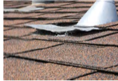
Typical Deficiency - Pipe jacks are damaged. Recommend installing new GSM roof jack and storm collar.
