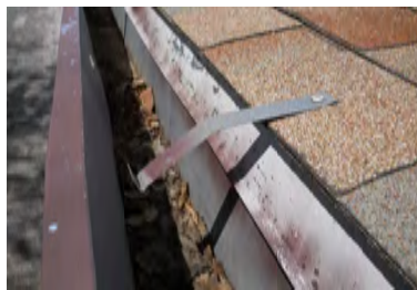
Typical Deficiency - Gutter brackets have been face fastened through asphalt shingle. Recommend removal and repositioning bracket. Repair asphalt shingles as needed.
