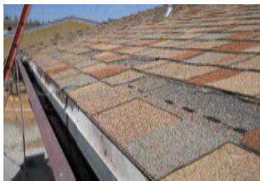
Typical Deficiency - Asphalt shingles are damaged and missing. Recommend replacing as needed.
