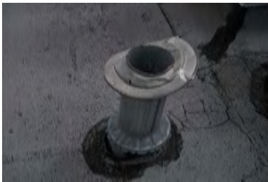
Typical Deficiency - Vent pipe is missing diffuser/ rain cap. Recommend installing rain cap and or replacement of vent.
