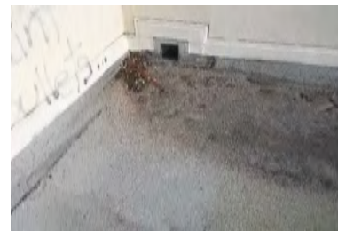
Typical Deficiency - Through wall scuppers should have debris screens. Recommend installation of gutter screens to promote positive drainage.
