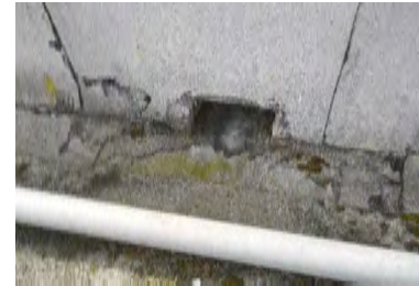
Typical Deficiency - Through wall scuppers should have debris screens. Recommend installation of gutter screens to promote positive drainage.
