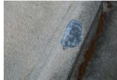
Typical Deficiency - Coating has begun to delaminate from perimeter coping cap. Recommend touch up as needed.
