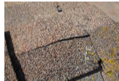
Typical Deficiency - Hip and ridge shingles are damaged and missing. Recommend replacing as needed.
