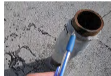
Typical Deficiency - Sealant at low slope roof jack needs to be replaced. Recommend re-seal and install storm collar.
