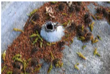
Typical Deficiency - Pipe jack at through roof penetration is damaged. Recommend repairing as needed.
