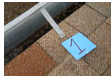
Typical Deficiency - Gutter brackets have been face fastened through asphalt shingle. Recommend removal and repositioning bracket. Repair asphalt shingles as needed.
