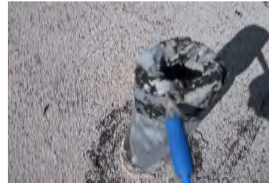
Typical Deficiency - Pipe jacks are missing sealant. Recommend application of flexible flashing self-adhered tape and or sealant, and install storm collar.
