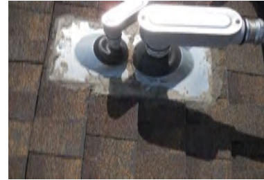
Typical Deficiency - Through roof penetrations has not been properly flashed. Recommend installing new roof jack and storm collar.
