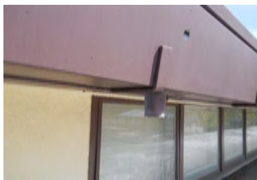
Typical Deficiency - Missing leader pipe. Recommend installation of leader pipe to divert water to lower roof.
