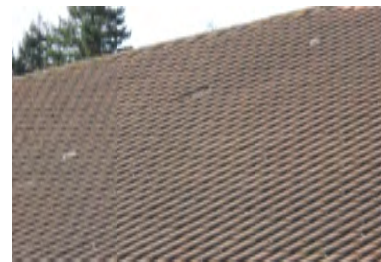
Typical Deficiency - Missing concrete S tile. Recommend replacement of all missing and or damaged tiles.
