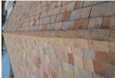
Typical Deficiency - Hip and ridge shingles are damaged and missing. Recommend replacing as needed.
