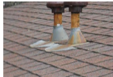
Typical Deficiency - Pipe jacks are missing band clamps and sealant. Recommend installing stainless steel band clamps, sealant, and install storm collar.
