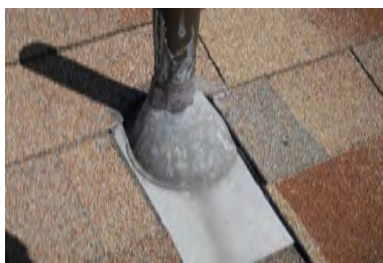
Typical Deficiency - Pipe jacks are missing sealant. Recommend application of flexible flashing self-adhered tape and or sealant, and install storm collar.
