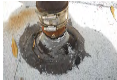
Typical Deficiency - Through roof penetrations do not appear to have proper low slope roof jack. Recommend installing proper roof jack and storm collar.
