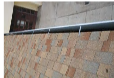
Typical Deficiency - Gutter brackets have been face fastened through asphalt shingle. Recommend removal and repositioning bracket. Repair asphalt shingles as needed.
