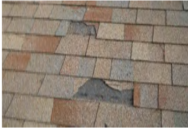
Typical Deficiency - Asphalt shingles are damaged and missing. Recommend replacing as needed.
