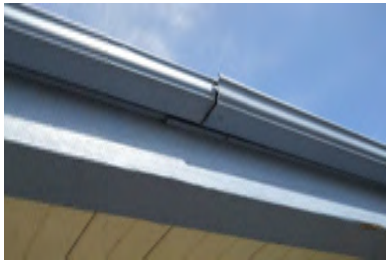
Typical Deficiency - Damaged gutter seam. Recommend repair as needed.
