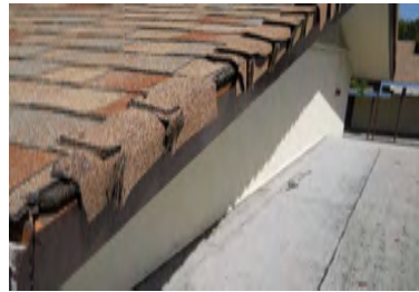
Typical Deficiency - Hip and ridge shingles are damaged and missing. Recommend replacing as needed.
