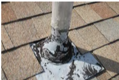
Typical Deficiency - Pipe jacks are missing sealant. Recommend application of flexible flashing self-adhered tape and or sealant, and install storm collar.
