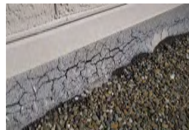
Typical Deficiency - Base flashings show signs of deterioration and cracking. Recommend application of silicone or acrylic coating to maximize usable life of existing built-up roof system.
