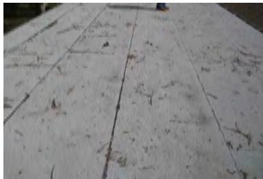
Typical Deficiency - Observed debris at field of roofing. Recommend clearing debris from all gutters, drains, waterways, and field of roof to promote positive drainage.
