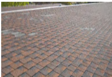
Typical Deficiency - Asphalt shingles are damaged and missing. Recommend replacing as needed.
