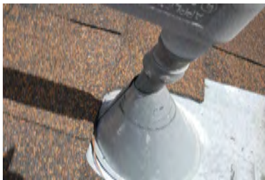
Typical Deficiency - Pipe jacks are missing sealant and or flexible self-adhered flashing tape. Recommend sealing, and install storm collar.
